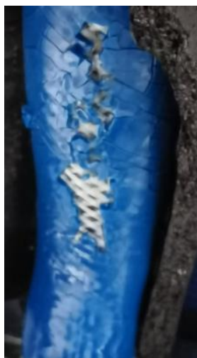
Figure 1: Degraded drain hose
