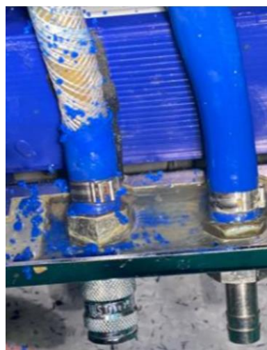
Figure 2: Degraded vs. intact blue colored hose
