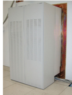
Figure 3. Filter Control Cabinet
