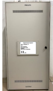
Figure 2. General Mains Distribution Unit
